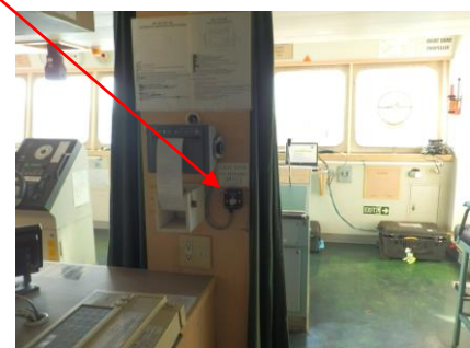
Figure 35. The Remote Reset Unit on chartroom starboard bulkhead.
