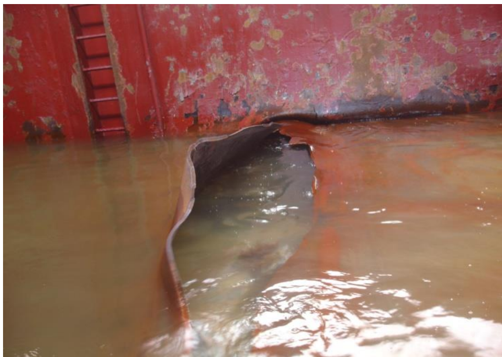
Figure 23. The crack at inner bottom plate of No 1 cargo hold as seen from inside .
