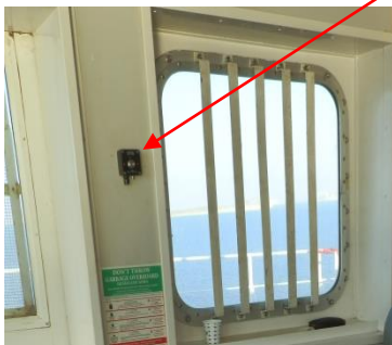
Figure 33. The Remote Reset Unit on starboard bulkhead.
